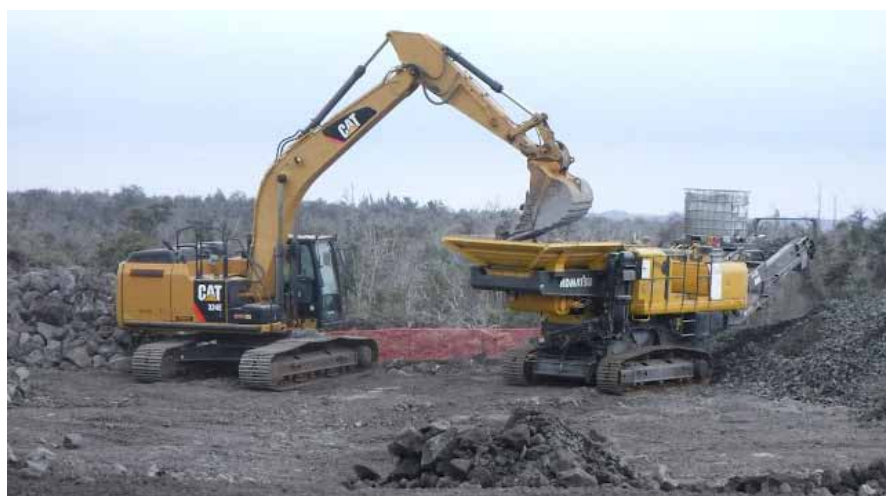
Views from where Iolani Blvd intersects the highway, showing earth-moving machines clearing an area of 'ōhi'a trees. The county owns a 21-acre lot; one acre is being developed for a temporary transfer station. A front-end loader drops a bucket-load of rock into a crusher that will reduce the size of the rocks to be used as a base for the new temporary transfer station in Ocean View.
