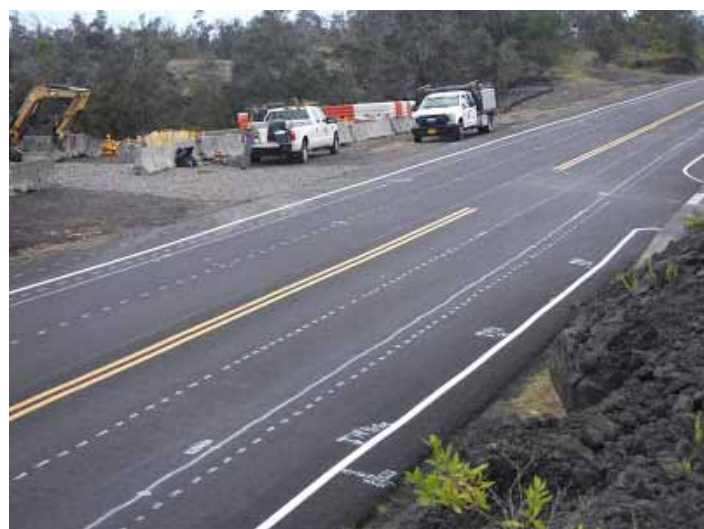
A plethora of spray-painted dotted lines, solid lines, and notes by surveyors indicates how Highway 19 will be widened and new lanes added to facilitate traffic turning onto the site of the new temporary transfer station in Ocean View.
