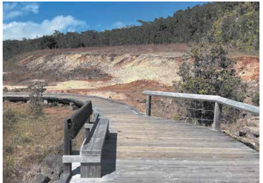
Degraded wooden boardwalk at Sulphur Banks Trail in Hawai’i Volcanoes National Park will be replaced through Dec. 12. NPS photo by Jessica Ferracane
