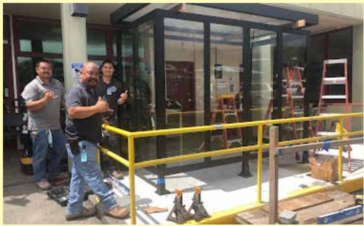
Curtis Higashi, Jay Taganas and Tyren Fukanaga-Camba erect a glass greeting and security station at the entrance to Ka'ū Hospital in Pāhala. Photo by Julia Neal
